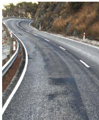
Figure 4. Bleeding and flushing on Category 2H curve
