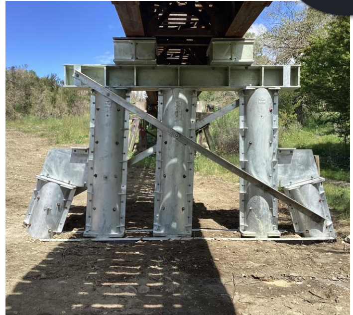
After: fully entombed bridge piers
