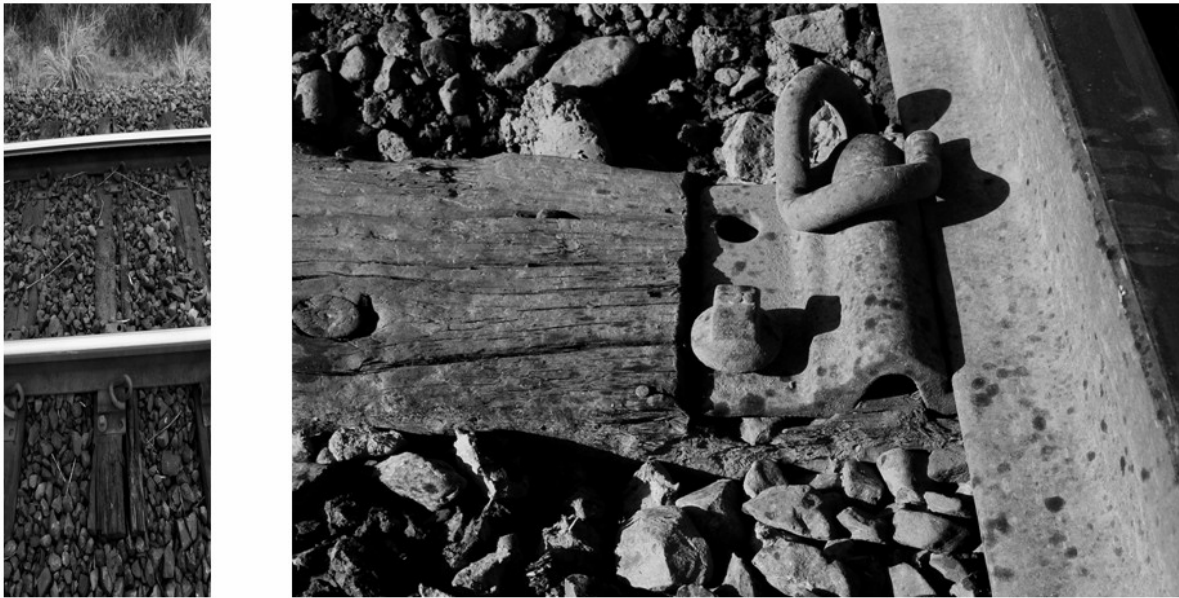
Figure 3.2 – Left: TPR sleeper with a large split running down its length. Right: bedplate supporting the rail cutting into the top of the TPR sleeper.
