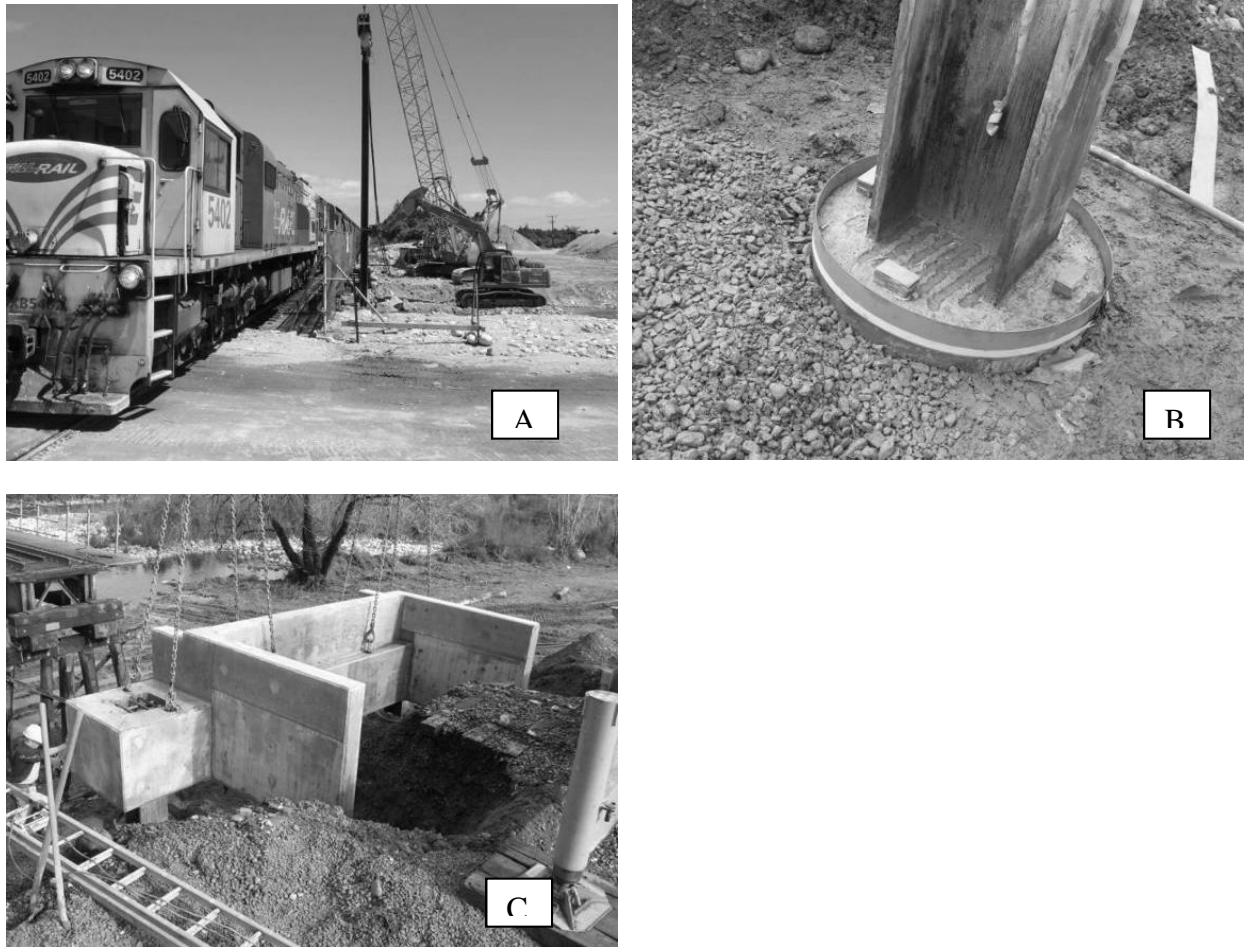
Figure 3.5 – Top Left (A): ‘H’ Pile being driven. A digger holds the pile in the correct position while a crane with driving gear installs the pile. Top Right (B): An installed ‘H’ pile after the concrete cylindrical collar has been formed. Bottom (C): a concrete pre-cast cap being lowered onto the ‘H’ piles during a rail shut down. In this example the cap also incorporates bridge abutment wing walls.
